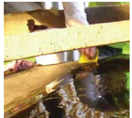
After Repair: Belt flap cut down, Devcon Surface Conditioner and R-Flex applied to belt.
